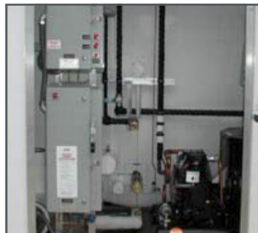
Electrical panels inside control cabinet for refrigeration system and optional pressure build vaporizer.
